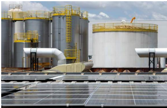
Solar array at Stepan's Salto Brazil site, supplying 100% of the energy for operations
