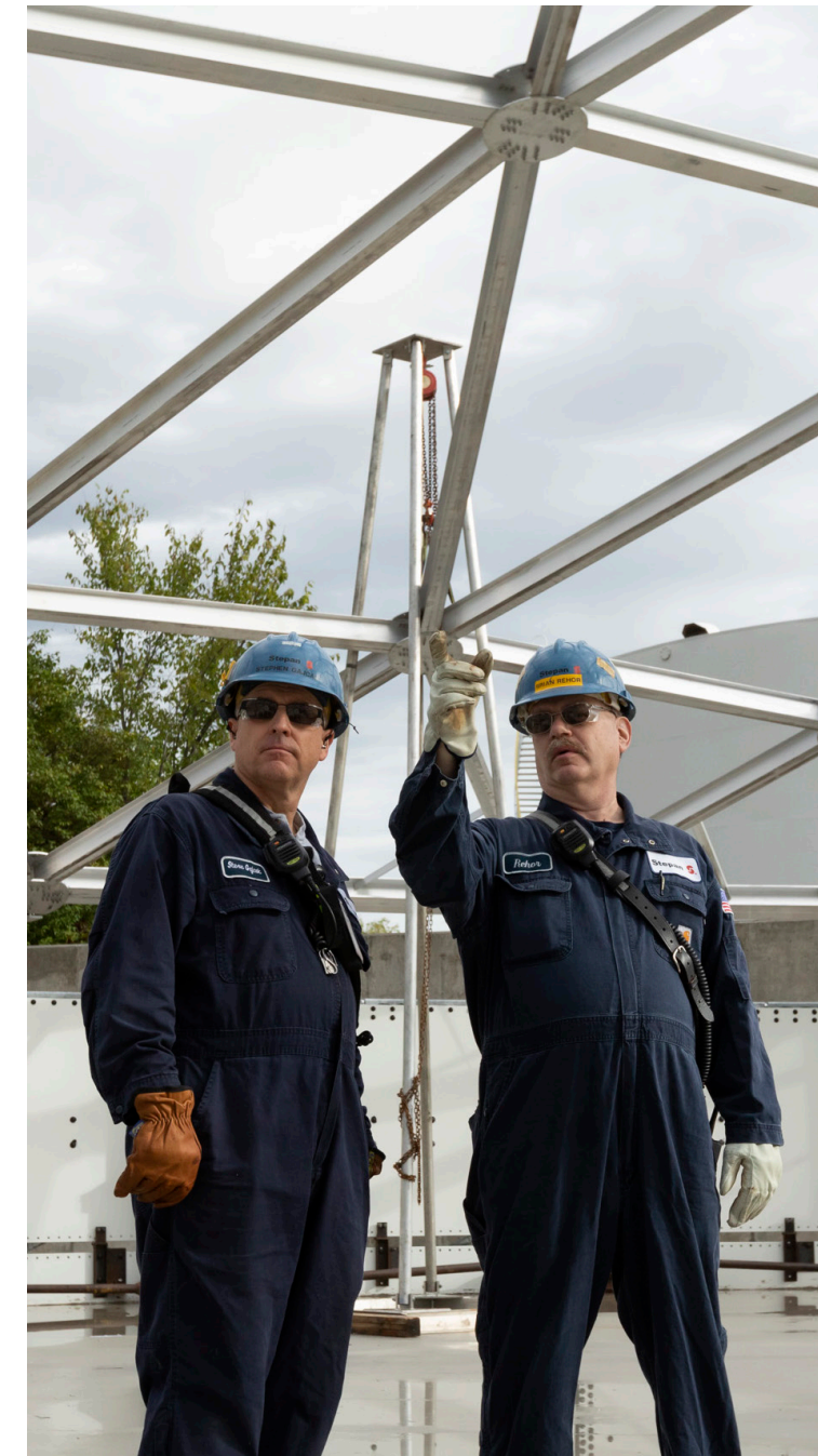
Steve Gajcak, Senior Construction Manager (left) and Brian Rehor, Production Shift Leader (right), Millsdale, Illinois
