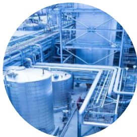
Stepan Fermentation Plant Lake Providence, Louisiana
