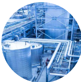
Stepan Fermentation Plant Lake Providence, Louisiana
