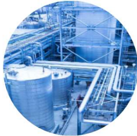
Stepan Fermentation Plant Lake Providence, Louisiana
